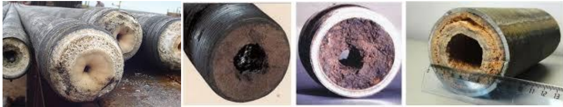
Figure 1 – Condition of pipes affected by ARPS complications
